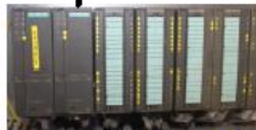
Automate Eclairage IP: 192.168.73.14
